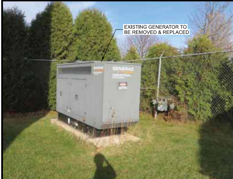
C EXISTING GENERATOR
