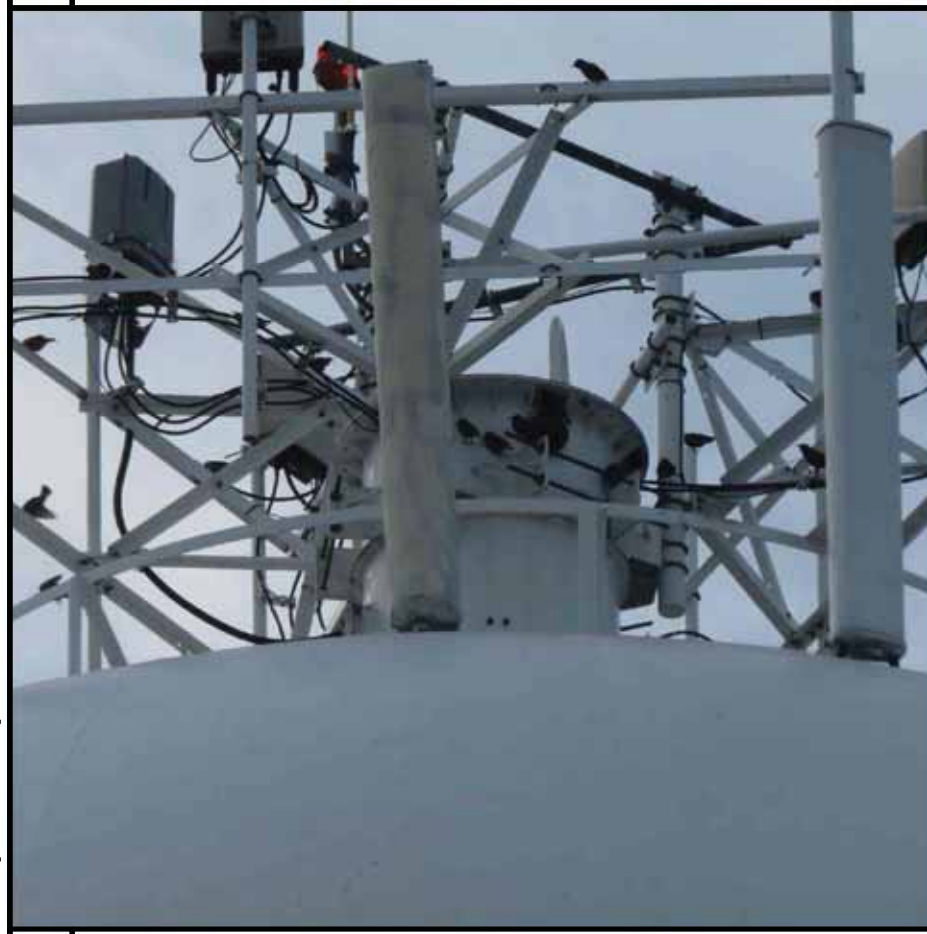
D TOP OF TOWER COAX PORT
