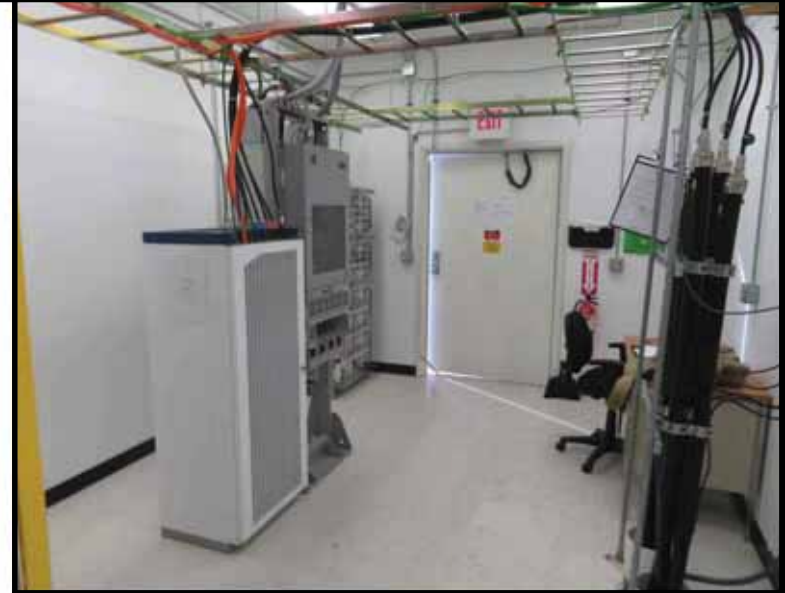
C EXISTING LTE EQUIPMENT CABINET
